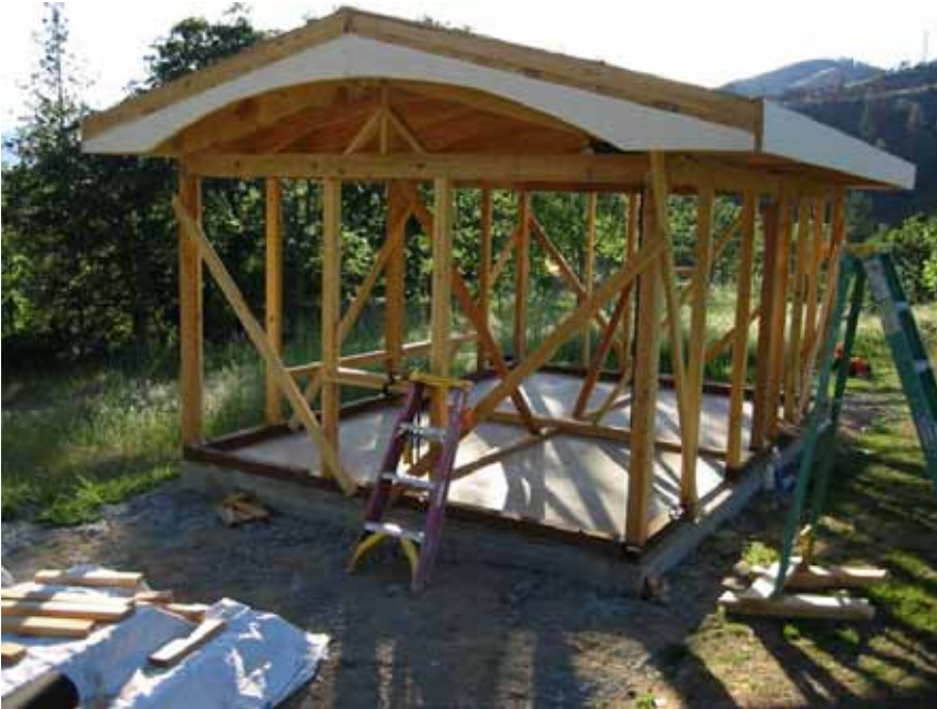
2 X 4 braces hold the walls plumb until bales or mesh are installed
